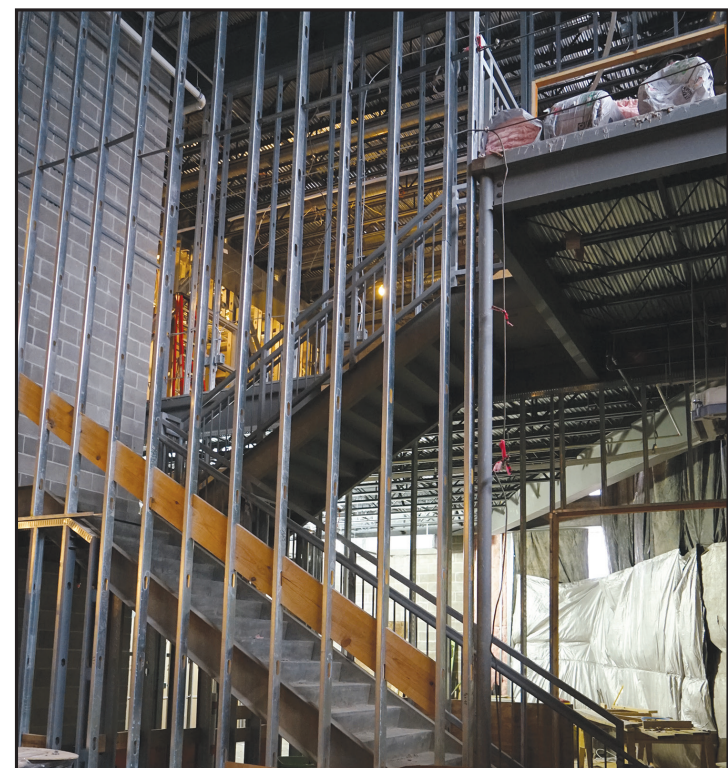
Photo courtesy of Lindenwood Public Relations The new staircase under construction in the LARC.
