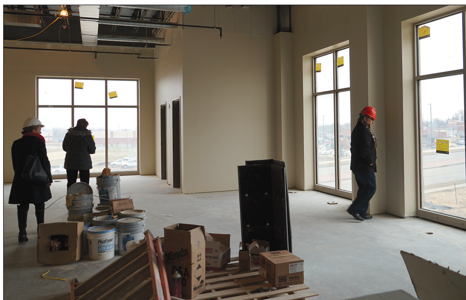
Photo courtesy of Lindenwood Public Relations Members of Lindenwood's administration take a tour of the construction happening in the LARC, which is scheduled to be built by next fall.
