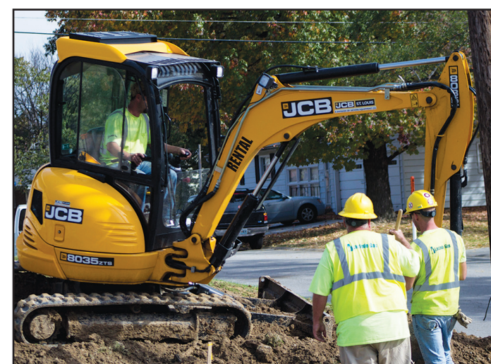
Photo by Kelby Lorenz St. Charles City workers dig up the gas main by Droste Road.
