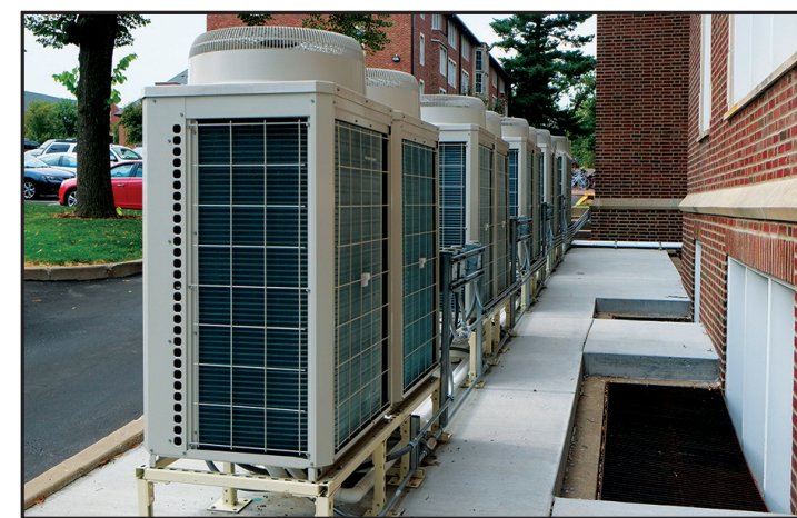
Photo by Nao Enomoto Within a years time, Sibley may get air conditioning units like these recently installed at Irwin Hall.
