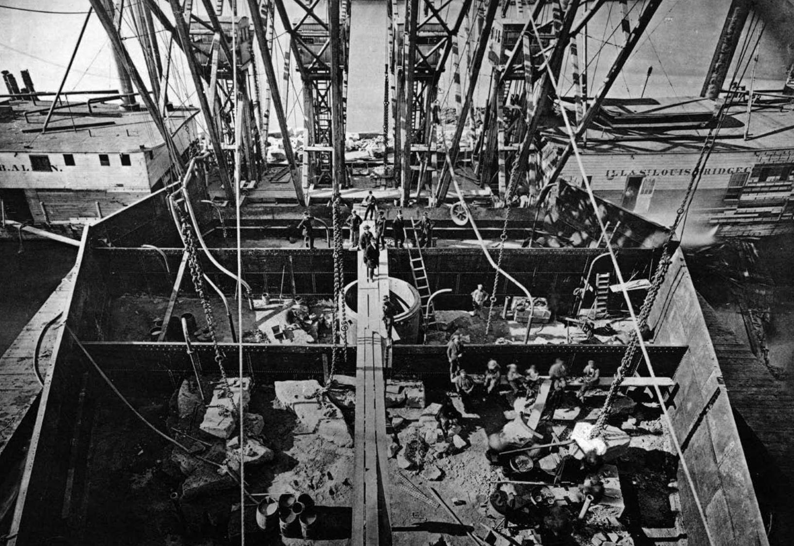
Construction of caissons allowed Keystone Bridge Company, the construction company hired to build Eads' design, to reach all the way to bedrock below the riverbed. Here, workers are sinking the east abutment, laying masonry on the floating caisson. (Photo: C. W. Woodward, A History of the St. Louis Bridge , 1881, Western Historical Manuscript Collection)
