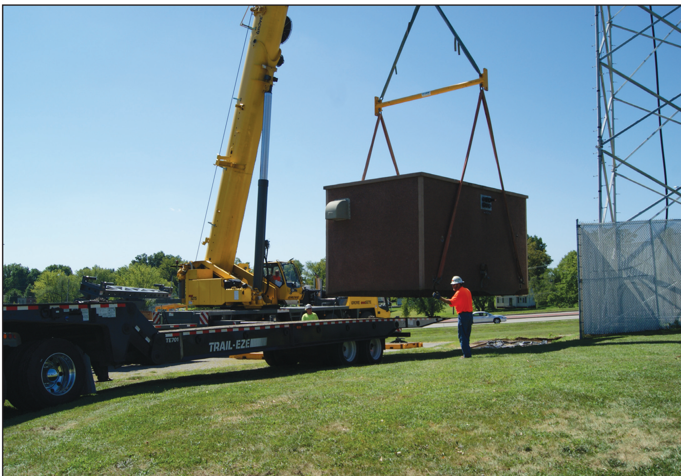
Workers use a crane Aug. 16 to lift the KCLC radio building from its old position to its new location behind the softball fields. Communications Dean Mike Wall said the move will help cell phone company AT&T provide higher quality service to students. In addition, the station will work on 50,000 watts (up from 35,000 watts), which will improve the quality of the signal. The building weighed approximately 60,000 pounds.
