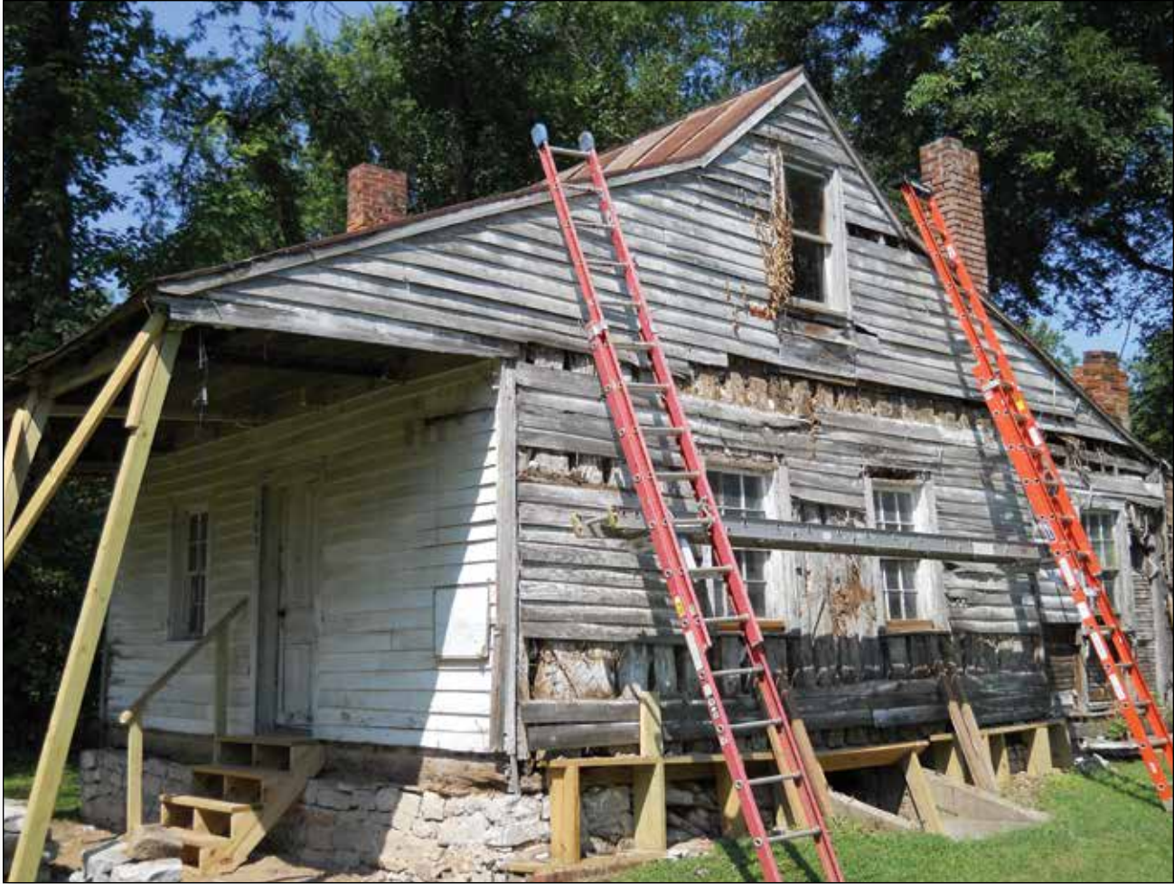
Lalumandiere House, 801 S. Gabouri Street, c. 1829, undergoing restoration. The vertical logs are visible in places where the siding is missing. (Image: Courtesy of the Author)
