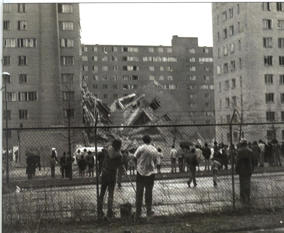
By the late 1960s, Pruitt-Igoe had become a symbol of violence and decay in high-density public housing. The federal government authorized razing the complex in 1971; the buildings were imploded starting in 1972, with destruction completed in 1976. (Image: Missouri History Museum)
