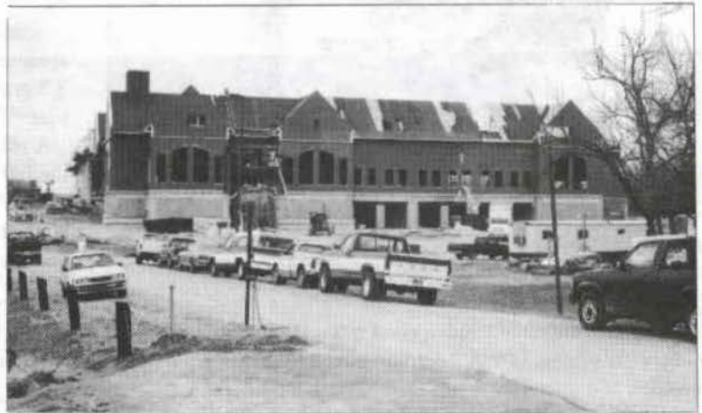
The Lindenwood College Performance Arena is taking shape on the back part of the campus. It is scheduled to open in the fall.
