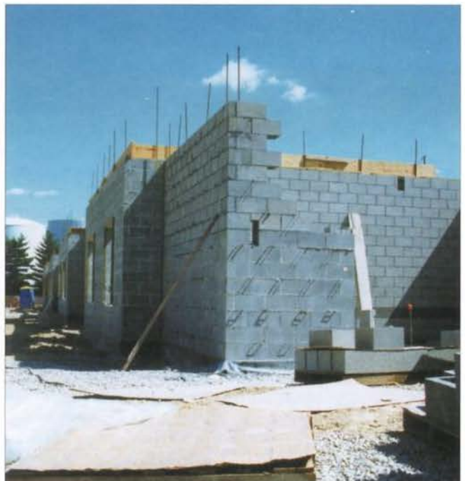
One of the two new residence halls in progress. Photo by Lindenwood student Tara Scotti.
