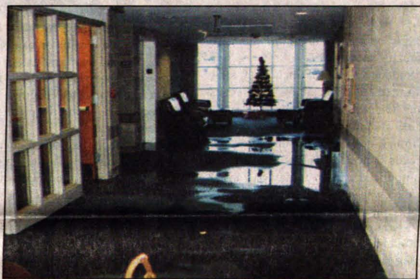
Courtesy photo Water spills into one of the floor lounges of Calvert Rogers dorm.
