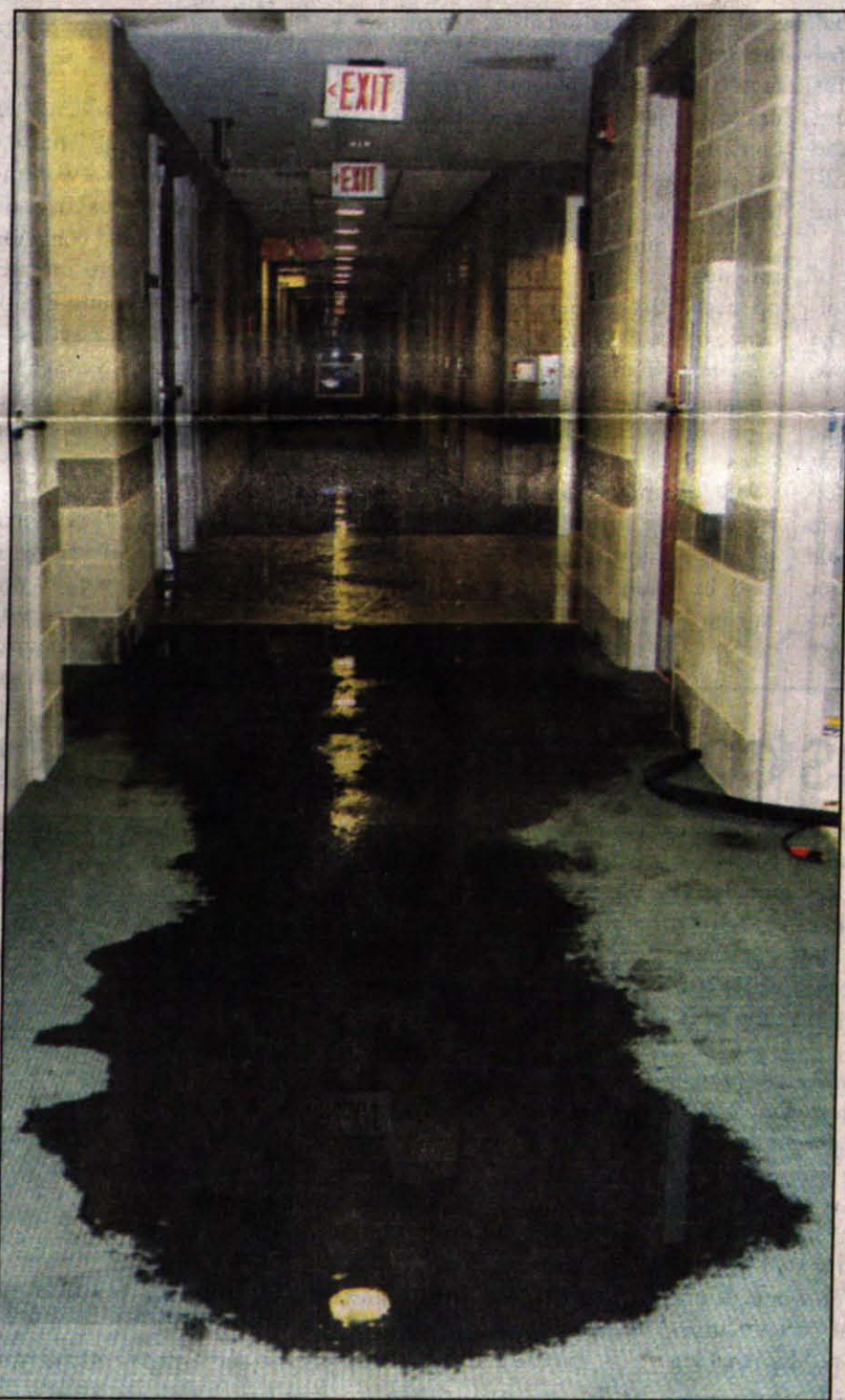
Courtesy photo Cold temperatures cause pipes in Calvert Rogers dorm to burst, causing water to flood the hallway. Residents said the first and fourth floors received the worst of the damage, and students were relocated into alternate housing until the damage was repaired.
