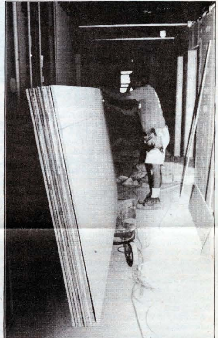
Workers renovating the 4th floor of Irwin Hall. The new floor will house 28 male students. Photo by Paul Butts ('79)
