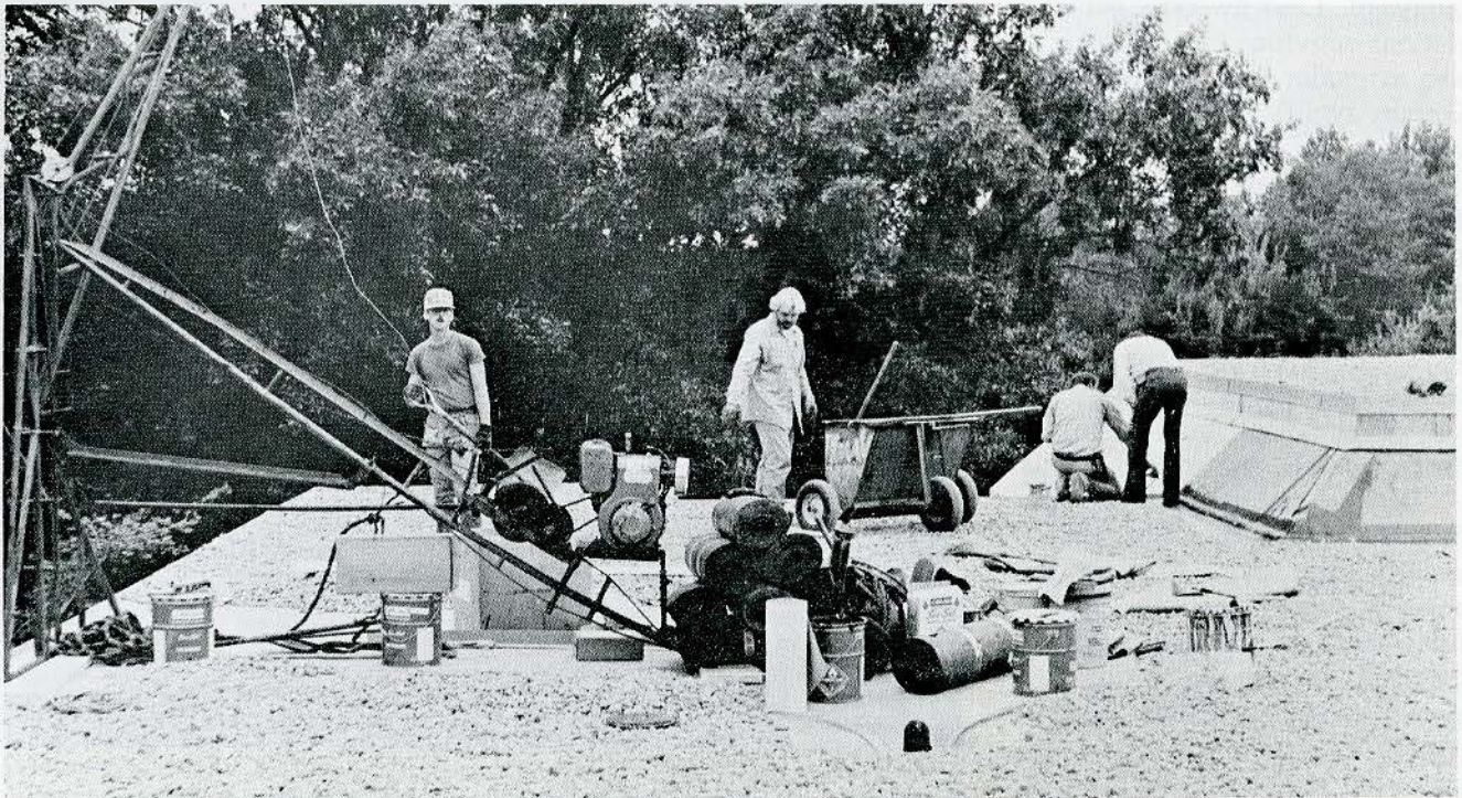
Nearly $45,000 was spent this year to construct a new roof on the Fine Arts Building, which contains modern studios, laboratories and classrooms for the Performing Arts Dept. The new roof will lead to cost savings in maintenance and energy of nearly $1,500 annually. With funds borrowed for the roof construction, the project is included in the $250,000 Capital Funds Campaign recently announced by the college.
