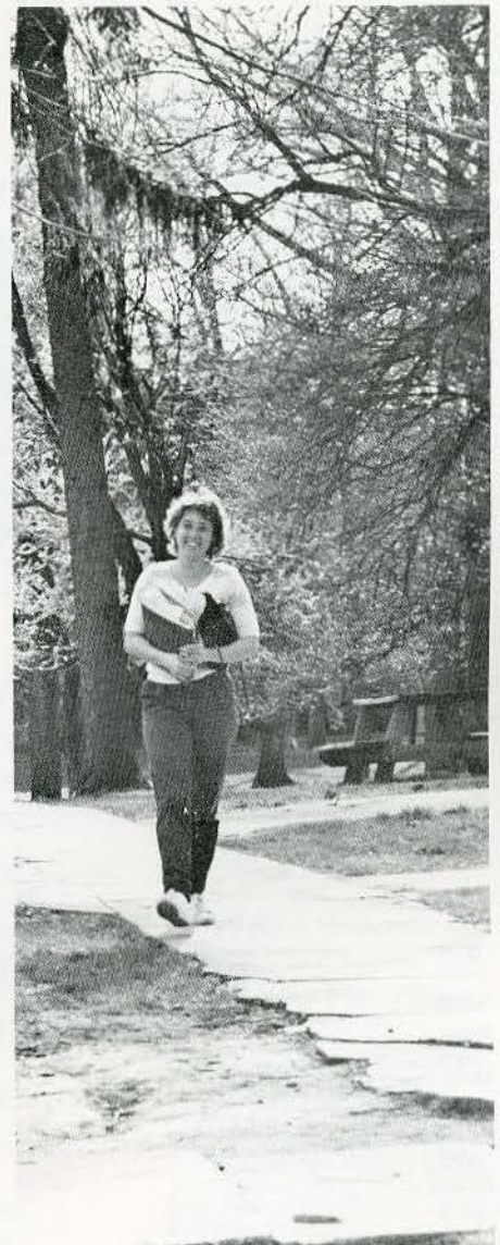
Nearly $12,000 is needed to repair decaying and cracked sidewalks found on the Lindenwood campus. The funding is part of $250,000 that will be earmarked to a capital funds campaign for renovation and repair of campus facilities.
