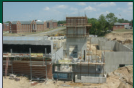
Construction on Lindenwood's Fine and Performing Arts Center is employing several hundred people
