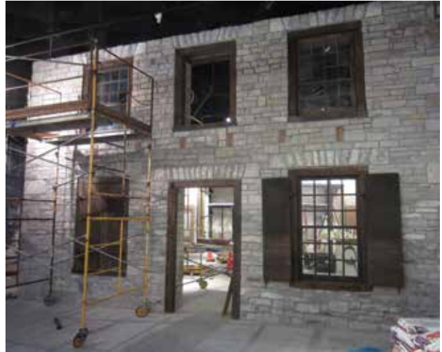
The east façade of the Old Rock House was reconstructed using all of the surviving original elements and the windows and shutters from the 1943 restoration. The exhibit will outline the building's use as a fur warehouse, a sail loft catering to western pioneers, and its years as a tavern and nightclub where African American artists performed blues music. (Image: National Park Service, Gateway Arch National Park)
